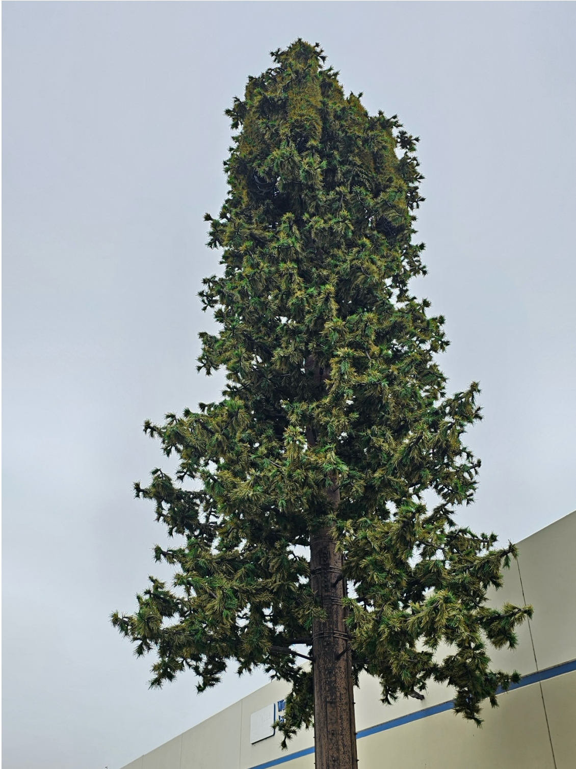
Tower and Equipment Cabinet – Current Conditions
