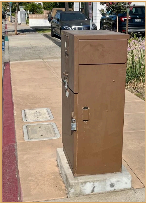
East (Side-Meter Pedestal)
