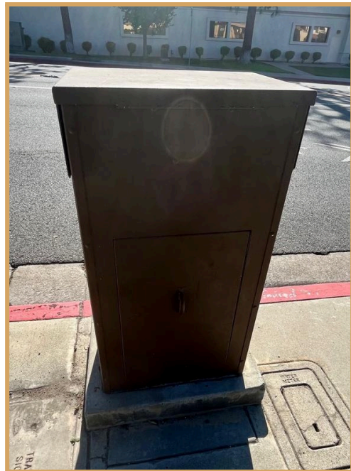
West (Back-Meter Pedestal)
