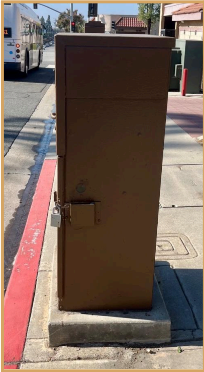
North (Side-Meter Pedestal)
