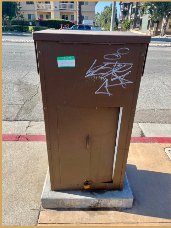
North (Back-Meter Pedestal)
