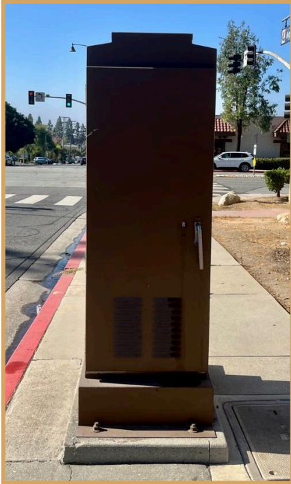
North (Side-Traffic Controller)
