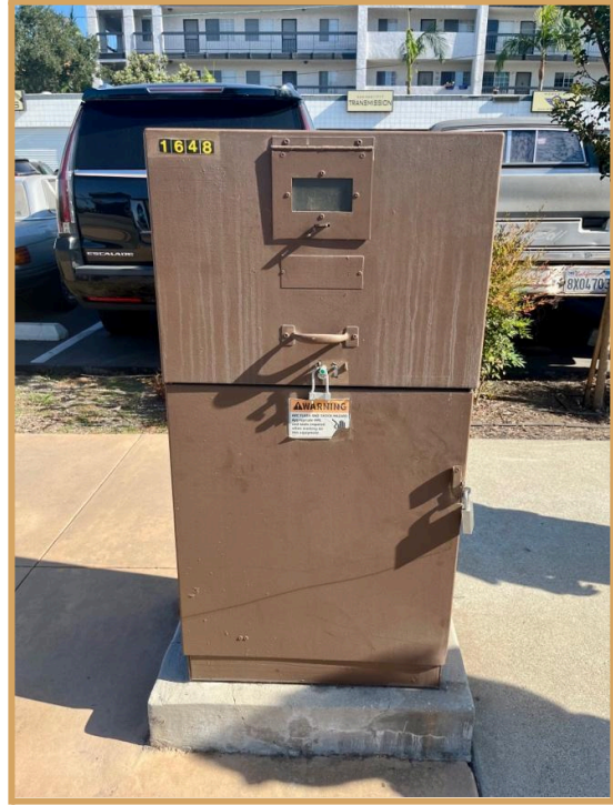
South (Front-Meter Pedestal)
