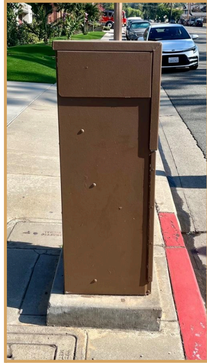
South (Side-Meter Pedestal)
