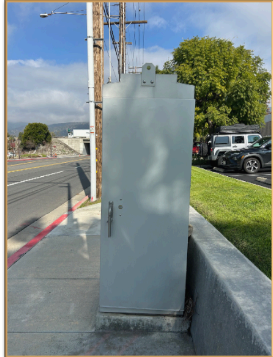
South (Side of Utility Box)
