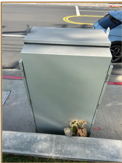
East (Back of Utility Box)
