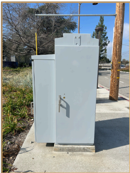
East (Side of Utility Box)
